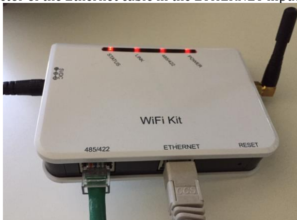
Figure 87 – Ethernet cable connected to the datalogger
