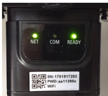
Figure 77- Irregular communication status between inverter and adapter
