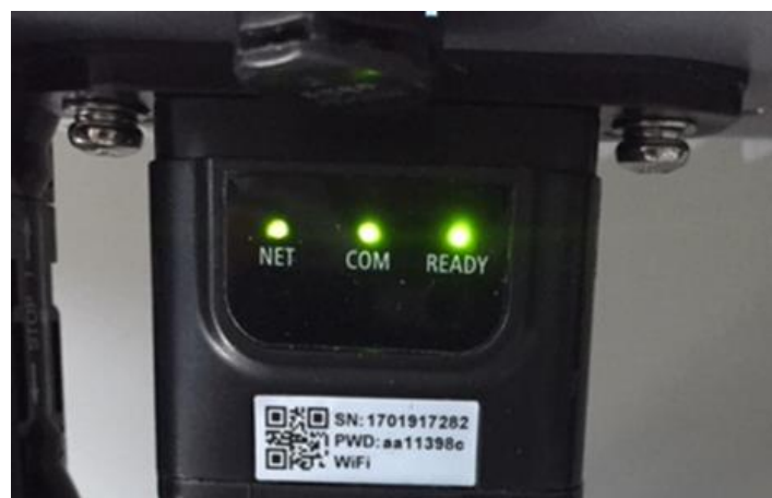
Figure 70 - Final status of LEDs
